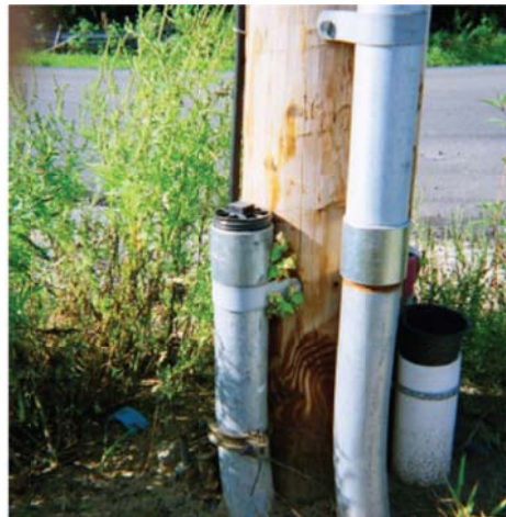
Spare Riser Sweep Spare sweep shall be bonded to down ground and capped at riser pole.
