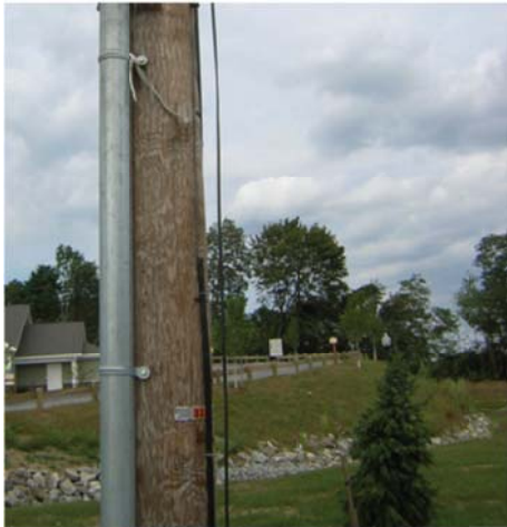
Riser Pole Bonding Rigid Galvanized Steel. Bond higher than 8' and at least 6" from top.
