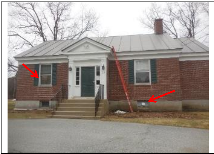
1. ACBM hard grey and hard tan caulking is present around the windows and vents.
