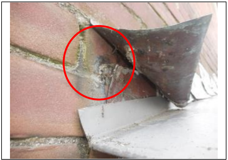
2. ACBM mixed mastics under the metal flashing between the bulkhead and the library building.
