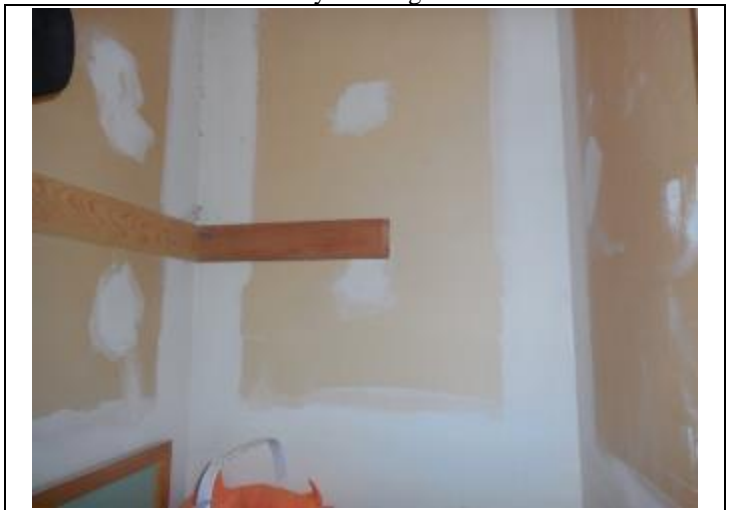
4. Gypsum wall board with joint compound containing trace chrysotile.
