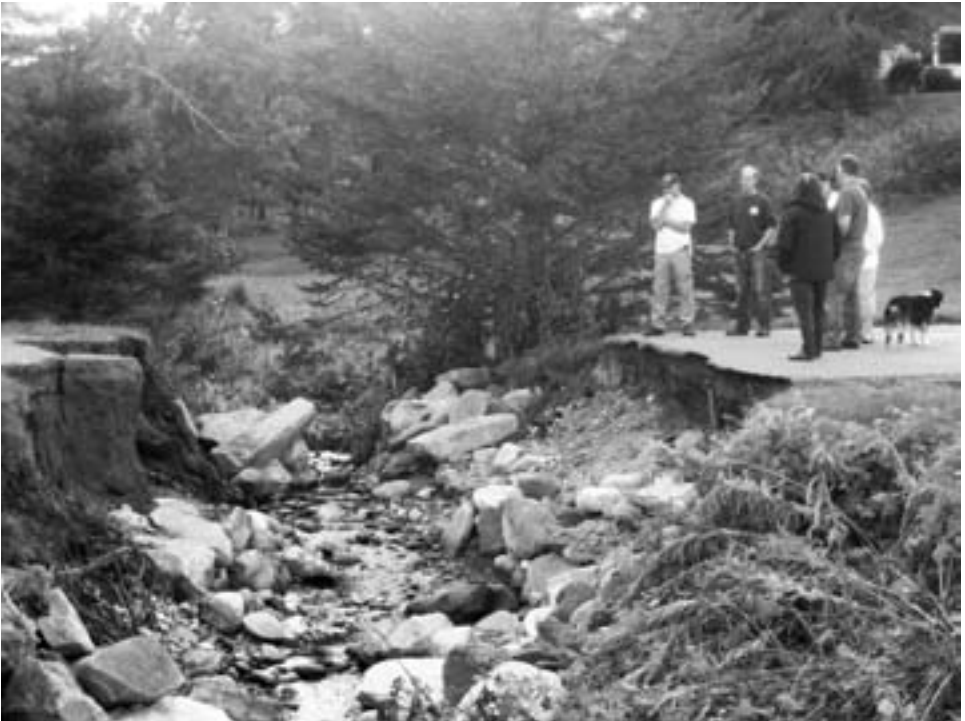
Selectboard surveys damage to Barker Road from tropical storm Irene Photo S. Halleran
