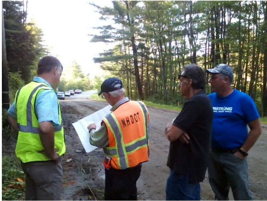
Reviewing the grade plans for Penniman Road prior to Paving Photo S. Halleran
