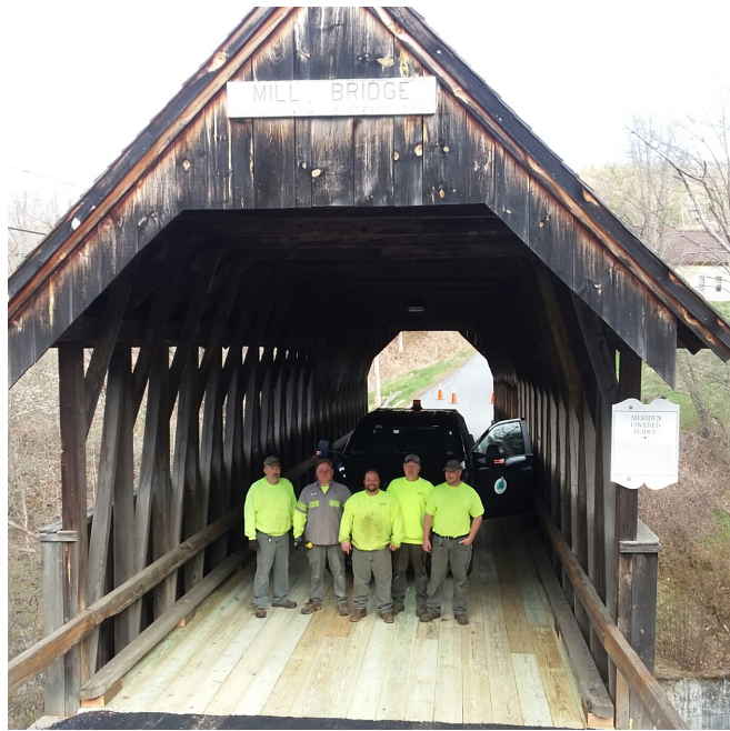
Meriden Covered Bridge 2020 (steel cleaned painted, new deck installed) Modern Protective Coatings Inc/Plainfield Highway Department
